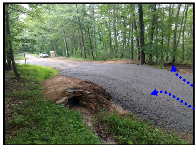
WITH GRADE BREAK (and associated crosspipe) – Interruption in slope redirects flow and guides water to a pipe inlet and a turnout.
