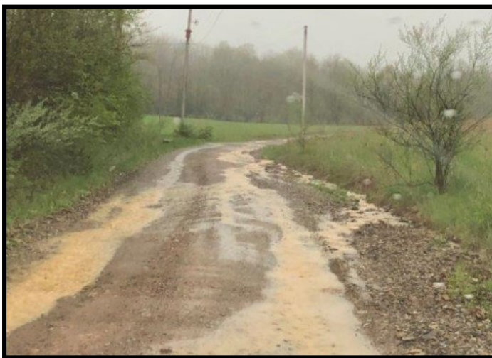
NO GRADE BREAK – Water flows on road causing excess erosion and aggregate loss.
